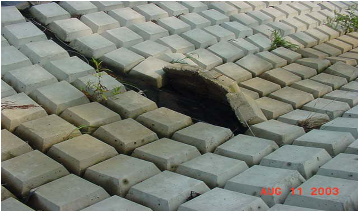
Photo 1 – Defective area South drain prior to making repairs
